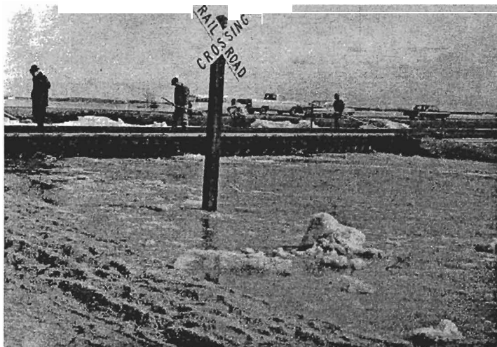
The Grivi Bridge was damaged in the Flood of 1966 (April). (photo courtesy of Milt Sather)
